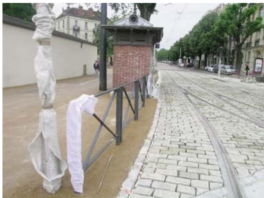
Barriers encourage pedestrians to cross the trackbed well downstream of the kiosk
