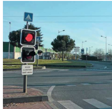
Photo 21: the R24 signal is installed at less than 2.20 metres since it is not a space used by pedestrians (source: Cerema)
