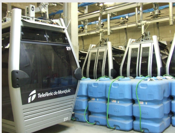
Barcelona: maintenance workshop for the gondola lift of Montjuïc. (Photo Anne Le Ruyet - CETE of Lyon)
